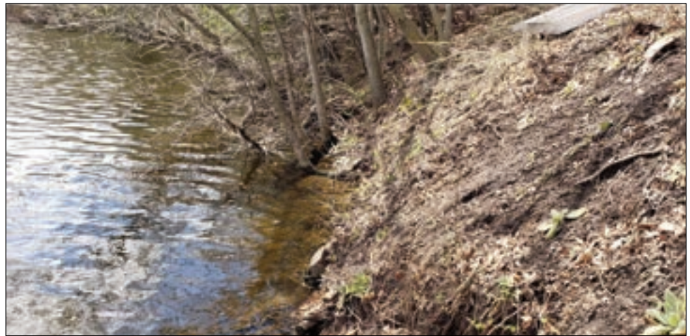
Shoreline where vegetation has been removed from slope and continued disturbance is leading to erosion on the slope and undercutting at the toe. Note the tree cut at the water's edge – if left to fall into the water, it would have provided shore protection. Also note the adjacent undisturbed area – no erosion concern there.
