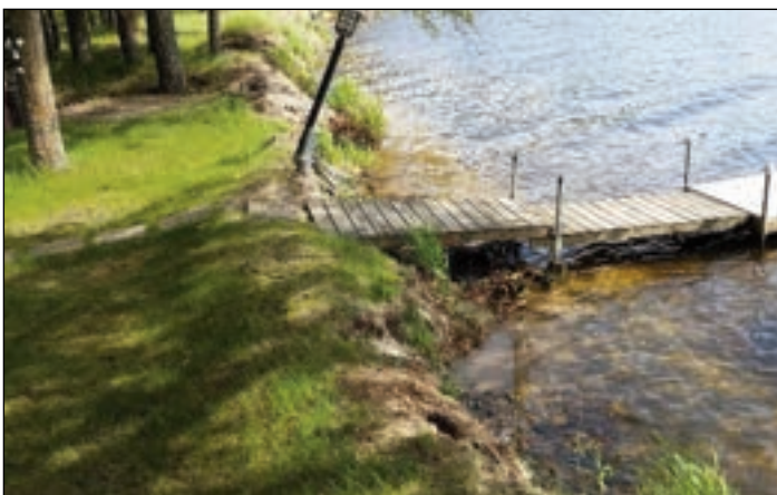
Eroding bank. Notice the lawn grass mowed up to the edge and the steep drop at the bank. Undercutting is very common in these situations. Regrading to a gentler slope & coir log is a good stabilization choice in this situation.
