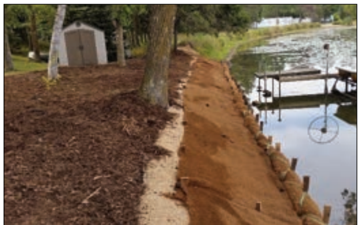
Regrading completed, coir log in place, erosion control blanket down. Now it is time for plants. Hundreds of native flowers, grasses, sedges, shrubs, and trees are options here – including low-growing plants. Notice how access is easier and the view can be improved.
